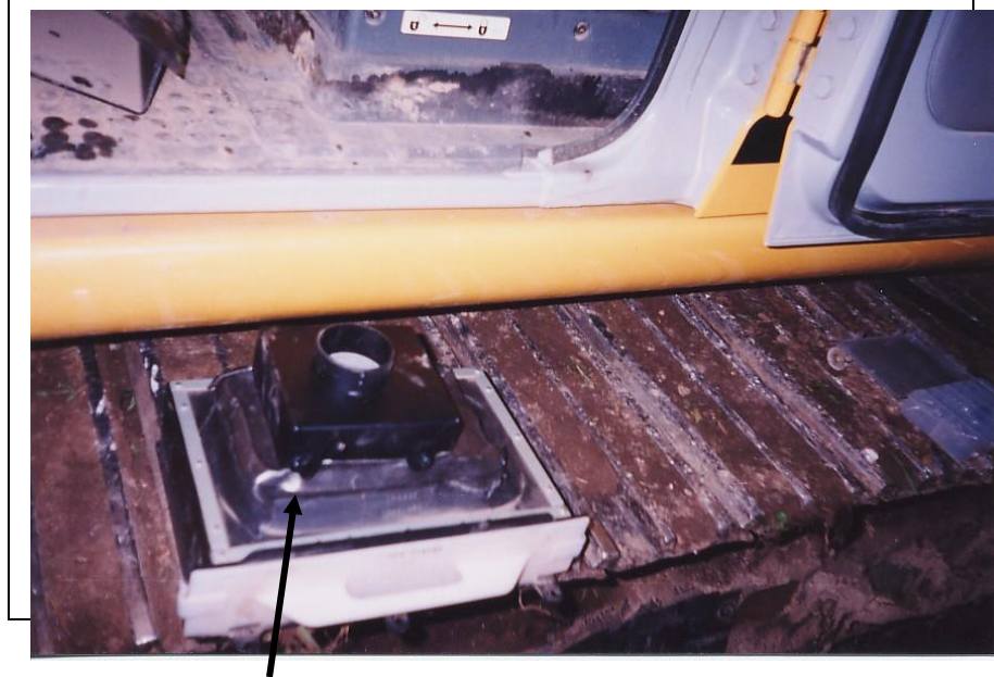
Outside air filter assembly with outside air intake box mounted and ready for reinstallation.
