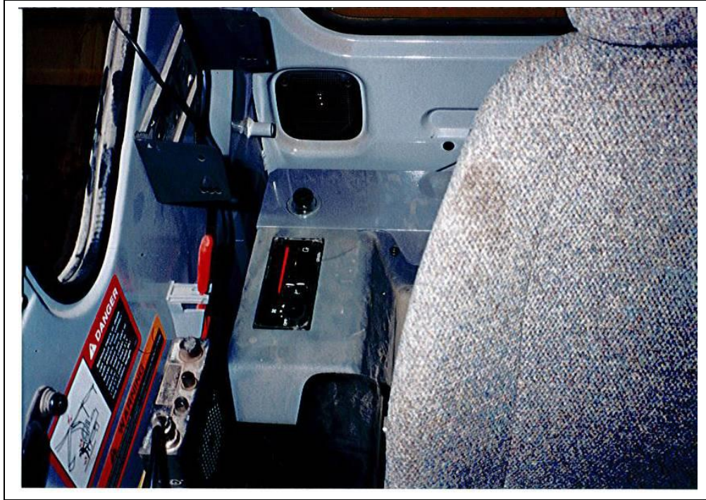
Another common area to mount the AC thermostat control.
